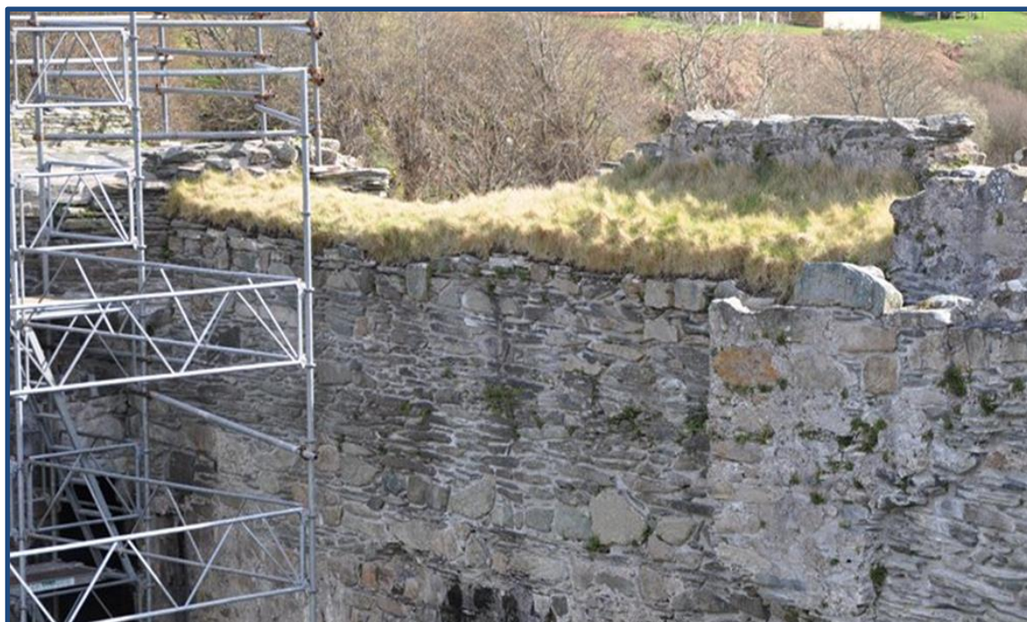
Figure 2. Castle Sween, Argyll. 'Soft capping' is considered a technically effective, as well as visually acceptable solution. Slow growing 'turf' is placed over an impermeable clay barrier to prevent water penetration to the open wallhead.
